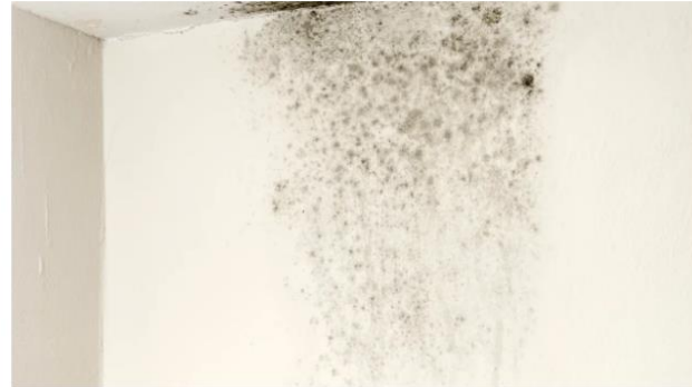
Mould is most common in rooms which produce moist conditions, such as kitchens and bathrooms (Photo: oneblue/light/Getty)
